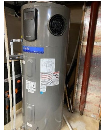
Heat Pump Water Heater
